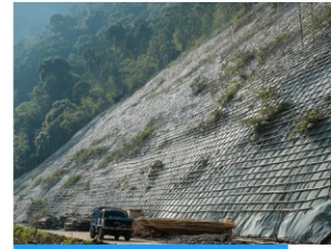
Rockfall Protection & Barriers
